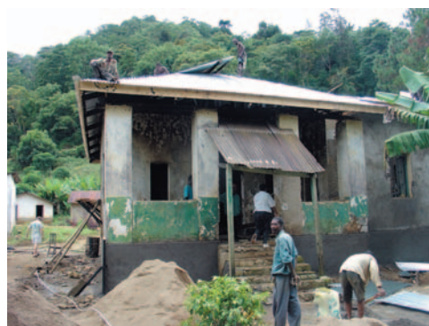
Many forest attendants houses are in a state of disrepair such as this building at Bunduki in the Uluguru Mountains. With support from CMEAMF, the house is being renovated. Photo by Neil Burgess
