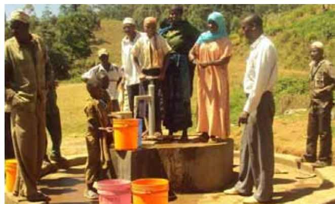
Water starts to flow from the new hand pump constructed by TFCG in Kwabosa Village in the West Usambara Mountains.
